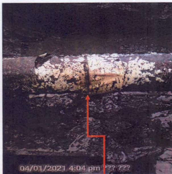
Fig B: Incident Facility shortly after exposure
